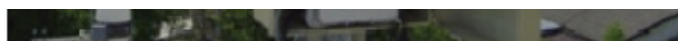
FIGURE 4: An installation example of a parabolic antenna and a wireless LAN unit to a steal pipe.
