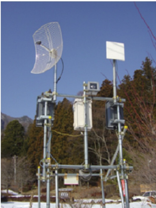
FIGURE 17: Yakushi Park relay station.
